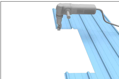
Use a nibbler to cut out the sheeting. NB! Do not use an angle grinder.
